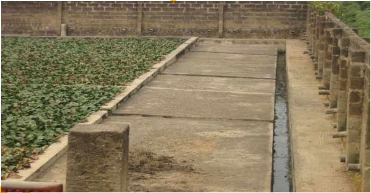
Plate 8: The Drainage System to Avoid Over Flow at the Sewage Treatment Work at University of Ibadan
