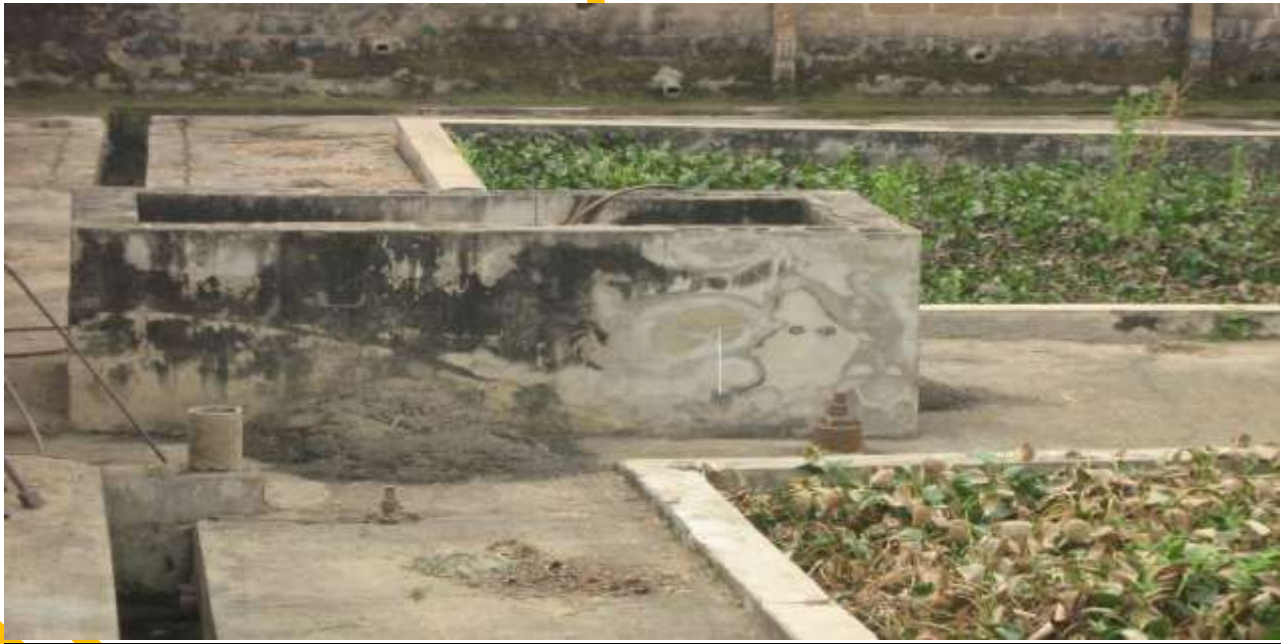
Plate 4: Side View of Distribution Chamber at the wastewater Treatment Plant at University of Ibadan
