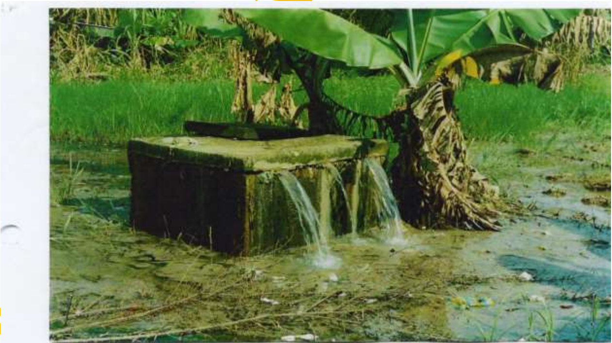
Plate 2: Overfilled Manhole at Wuse - Abuja
