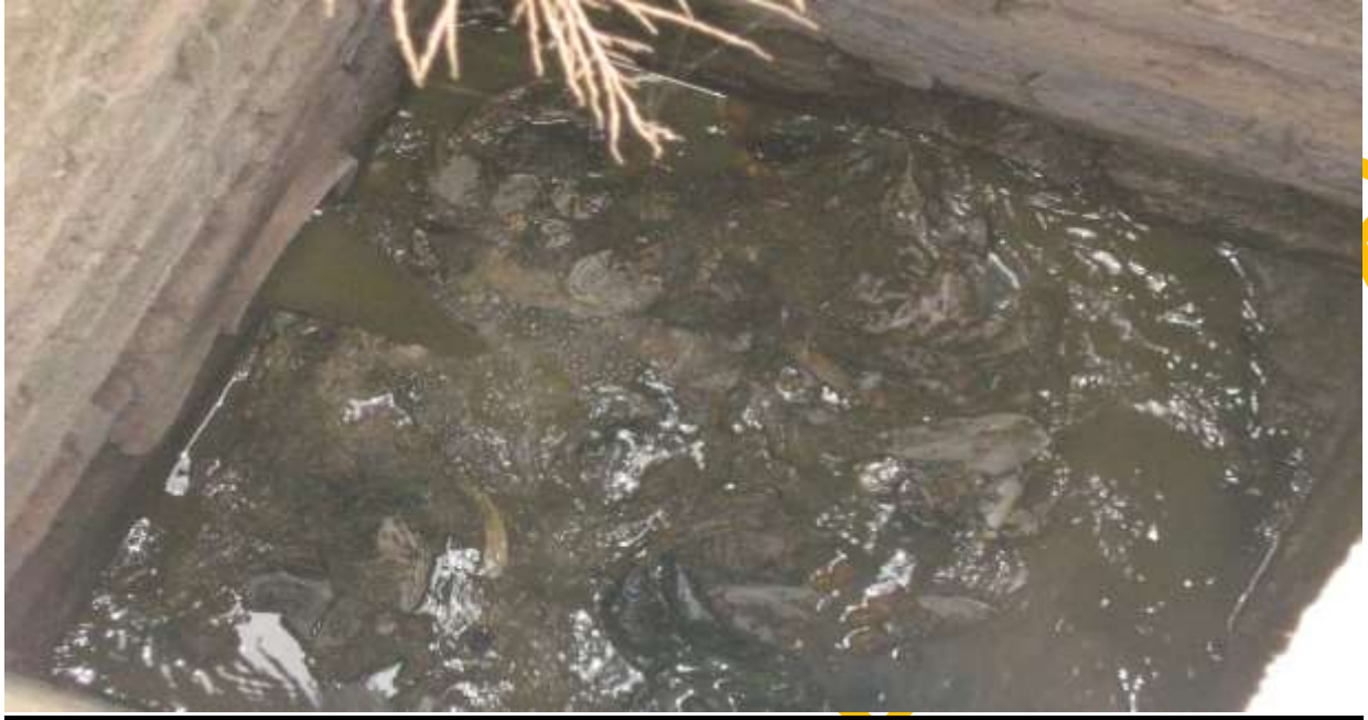
Plate 3: Inlet Chamber of the wastewater Treatment Plant at University of Ibadan
