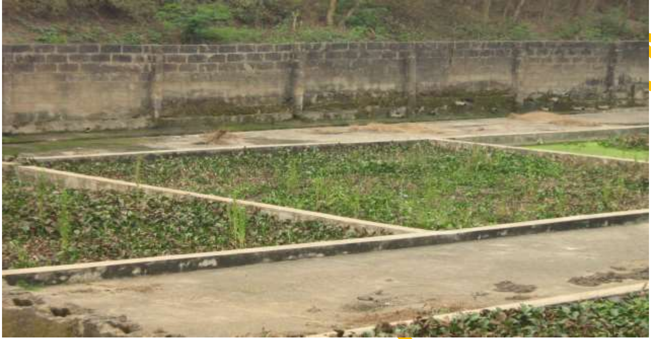
Plate 7: Closer View of a Chamber in the Sewage Works at University of Ibadan
