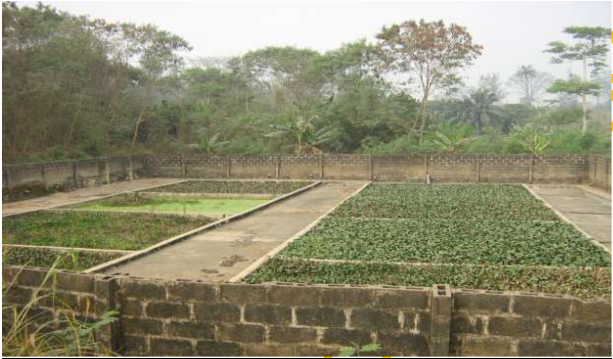
Plate 5: Frontal View of the wastewater Treatment Plant at University of Ibadan
