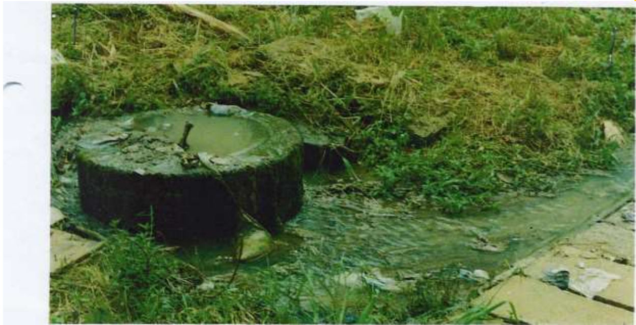
Plate 1: Blocked Manhole due to polythene bags at Gwarinpa District - Abuja
