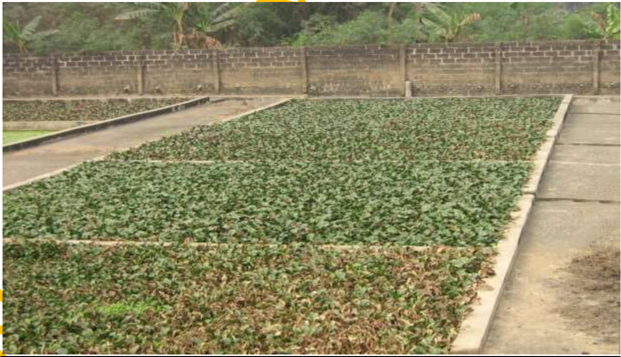
Plate 6: View of One Flow Line of the wastewater Treatment Plant at University of Ibadan
